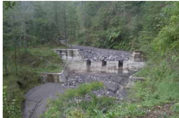
b). After debris flow occurrence
